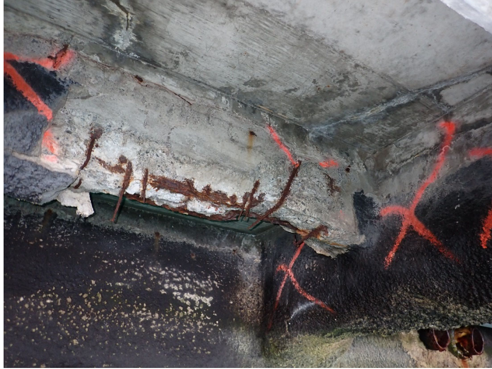
Photo 3: Typical Beam Spall
